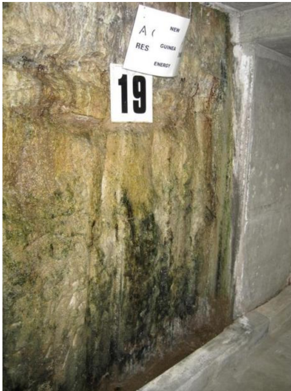
Figure 9 Groundwater seepage 2-10 Loftus Street
